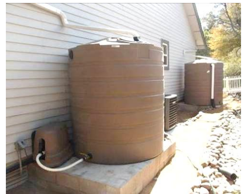
Fig 7 – Twin 650-gallon rainwater tanks beside Prescott home.
